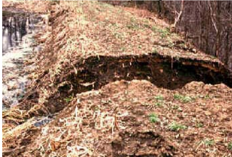
Figure 7-1 Example of embankment breach caused by overtopping of embankment.
