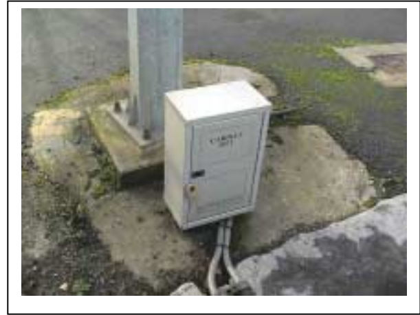
Plate 2.16 Gauge Control Box
