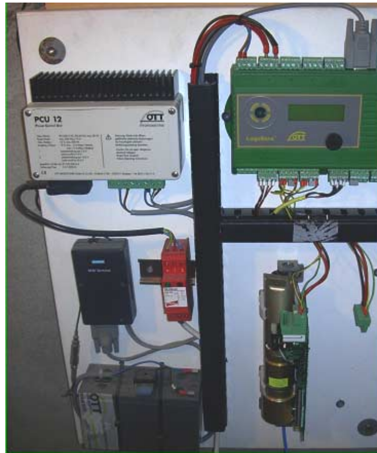
Plate 6.4 Tide Gauge Instrumentation (inside hut)
