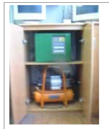
Plate 2.29 Processor and air compressor
