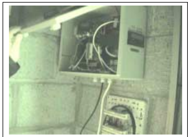
Plate 2.40 Gauge Control Box
