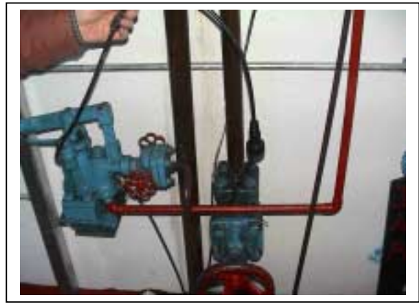
Plate 2.6 Cable End in Gate House
