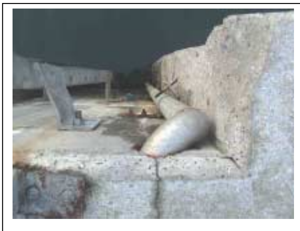
Plate 2.21 Pipe to Pressure Sensor
