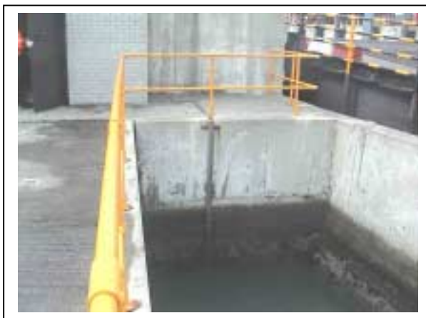
Plate 2.39 Rosslare Gauge Location (3)
