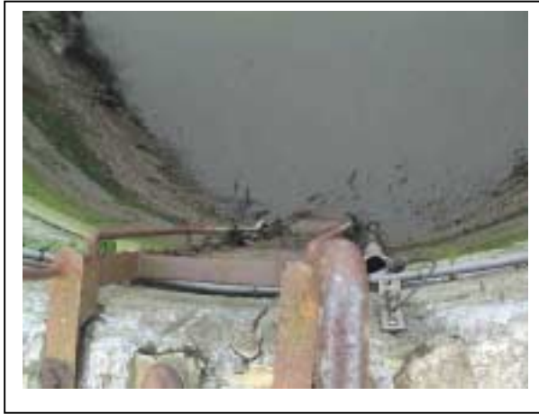
Plate 2.15 Pipe to Pressure Sensor
